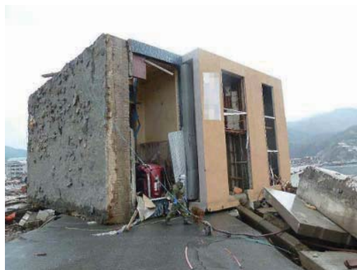
Photo 7.2-2 Overturning of a 3-story reinforced concrete building
